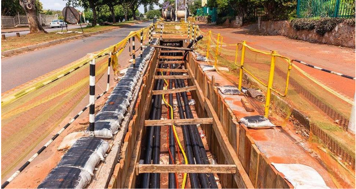
Figure I. 11: Câble HTA souterrain.
