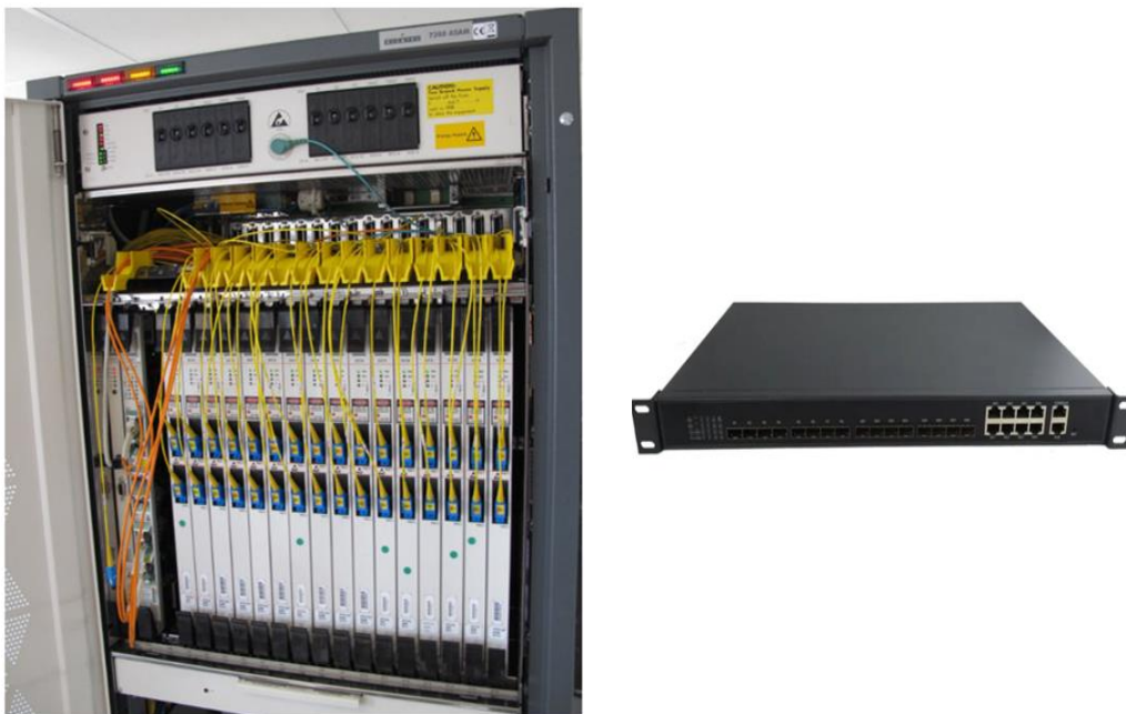
Fig 2.24: Optical Line Terminal (OLT) [7].
