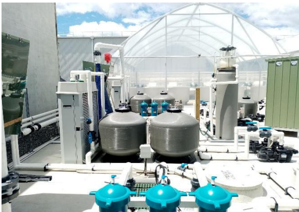
Pumping and Filtration Systems
