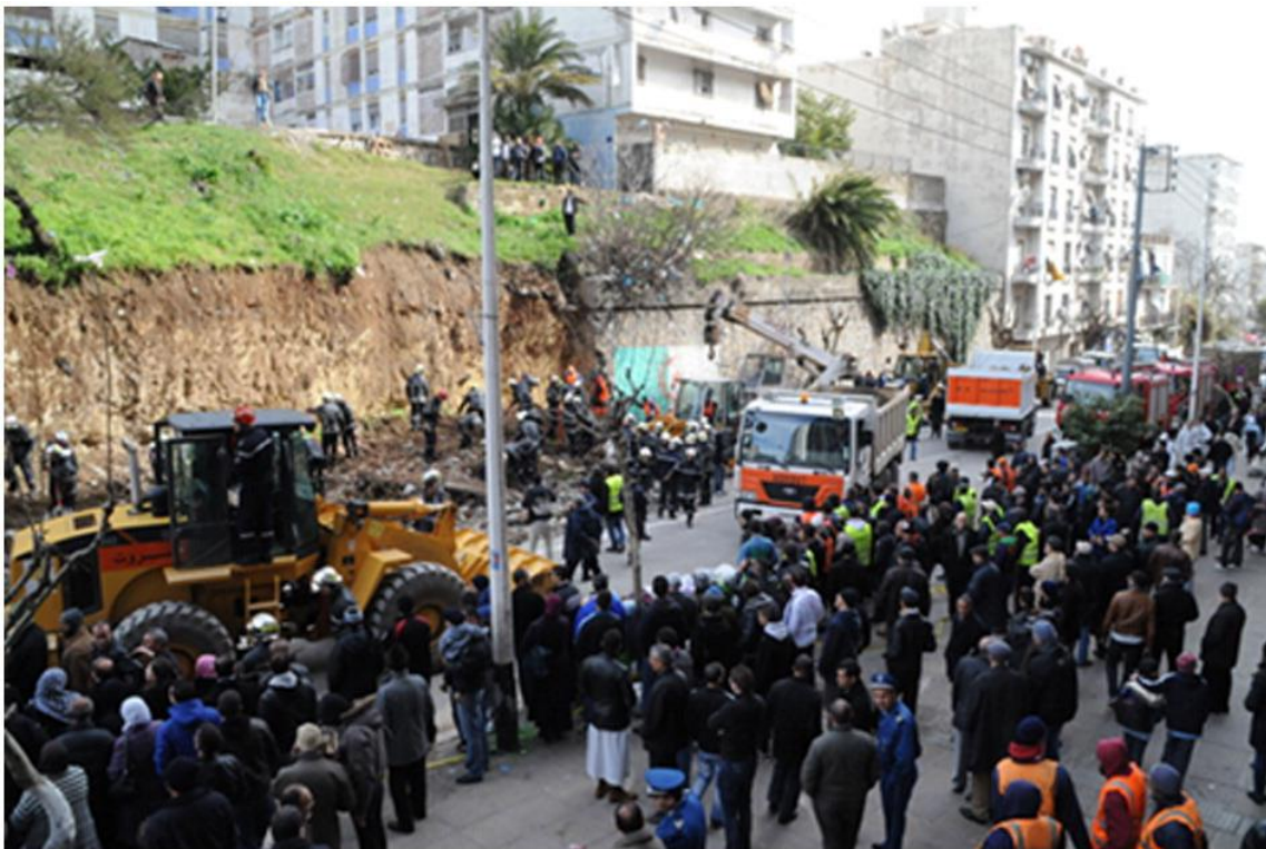
Figure 13: Retaining wall collapsed along Bougara Road after heavy rain in February 2013, (Abdallah , et al., 2014).
