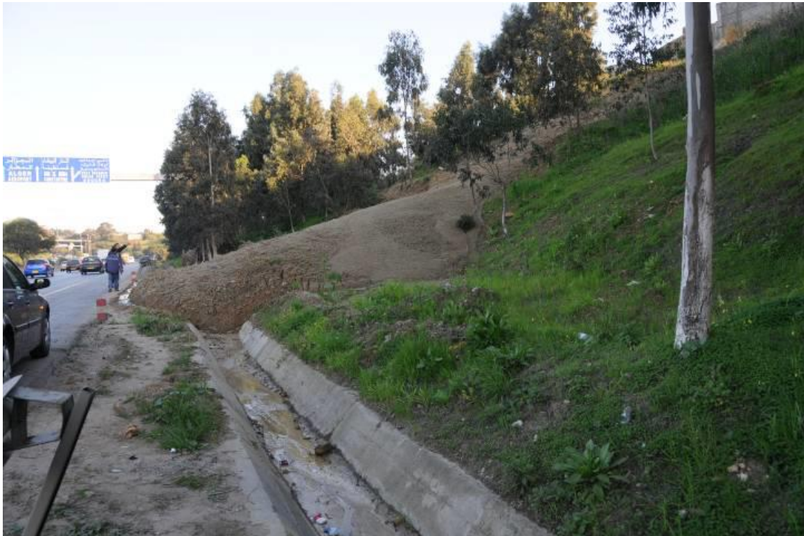
Figure 14: View of expressway and mudslide, source : ( ARAB Rabah, ZERMANI Messaoud, TABTI Saïd; 2009).
