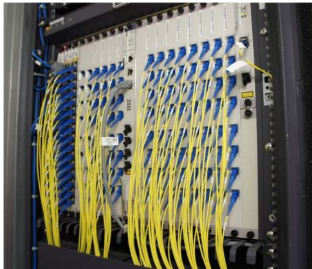
Figure.A.4 : Un OLT (optical line terminal)
