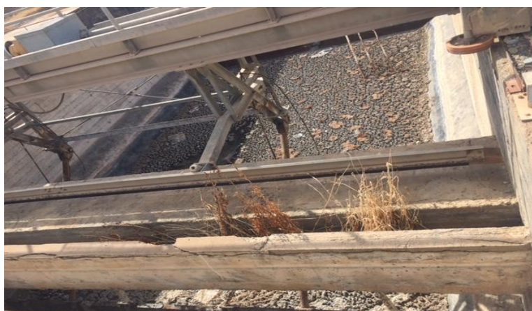
Figure III.4 : Bassin contenant la biomasse
