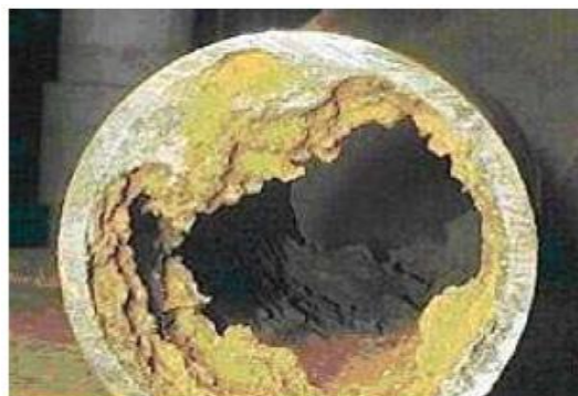
Figure .I.3: Corrosion Caverneuse
